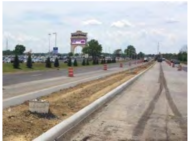
Kings Island Drive construction began in 2015. The project is a key component to the I-71/Western Row Road Interchange and a major gateway to the City.
