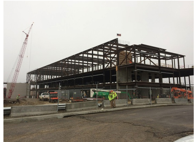
P&G Beauty Innovation Center continues construction at its existing business center 241-acre campus on Mason-Montgomery Road. The move to Mason will occur in the 2018/2019 timeframe.
