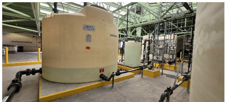
Photo 2: New pump/metering system for the application of corrosion chemicals.
