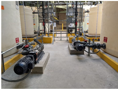
Photo 1: New bulk chemical feed system.
