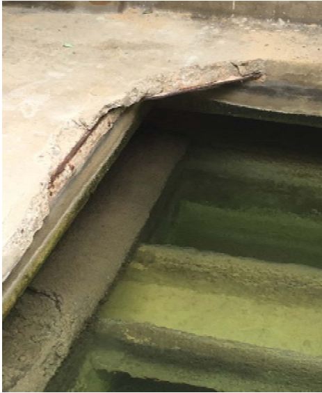
Photo 1: Photograph of the condition of the existing concrete walkways and support beams associated with the plant sand filter.
