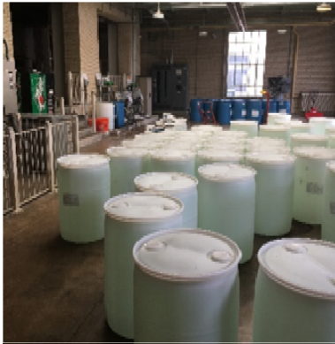
Photo 1: Existing Temporary Chemical Feed Configuration to be replaced by new bulk chemical feed system.
