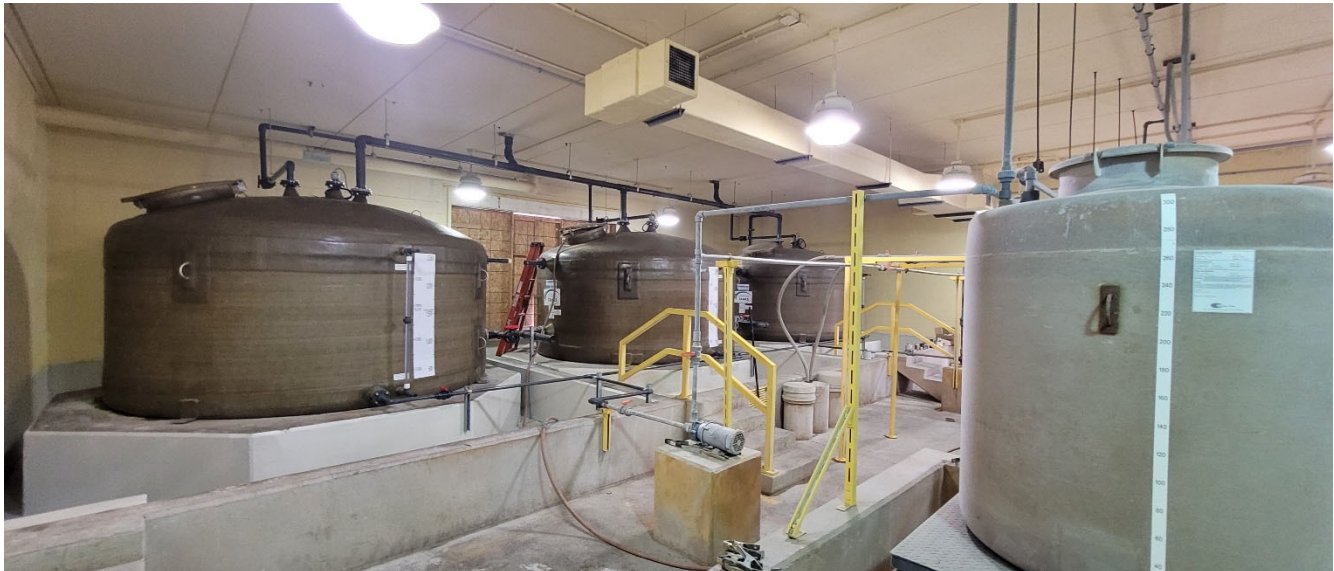
Photo 1: G-148 Fluoride System Replacement
